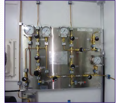
Gas Mixer Panel
