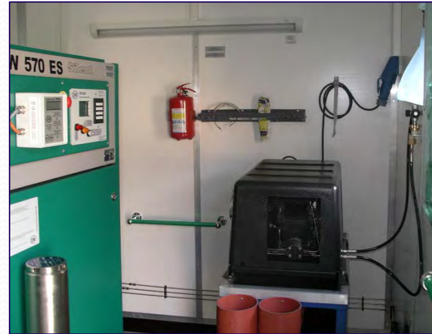
HP Air Compressor and HP O2 Booster
