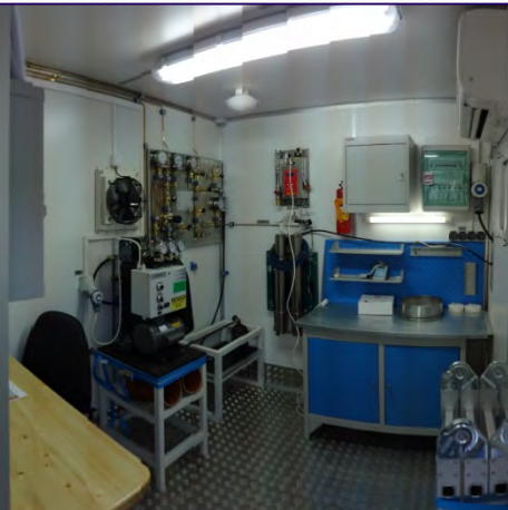
Gas Mixer Compartment
